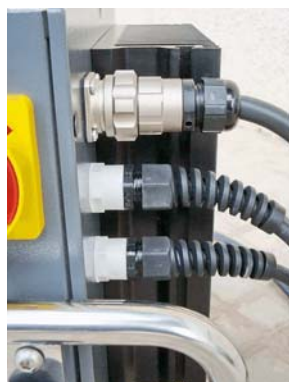
Figure 11a: Mains cable (plugged)
